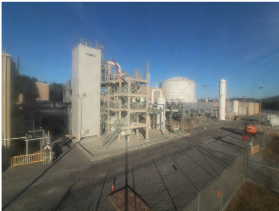
Figure 2: View of Liquefaction Site at the End of November 2025
