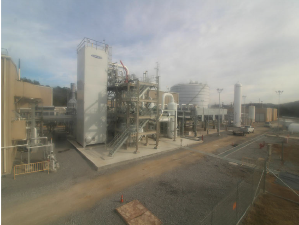
Figure 3: View of Liquefaction Site at the End of December 2025
