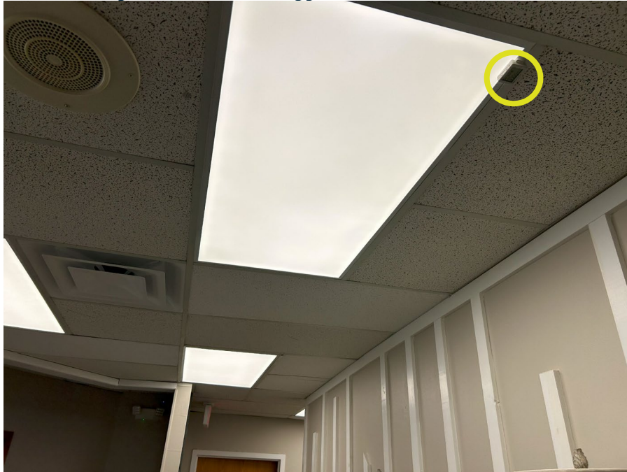
Figure 5-3. Installed Logger on Office Linear Fixture
