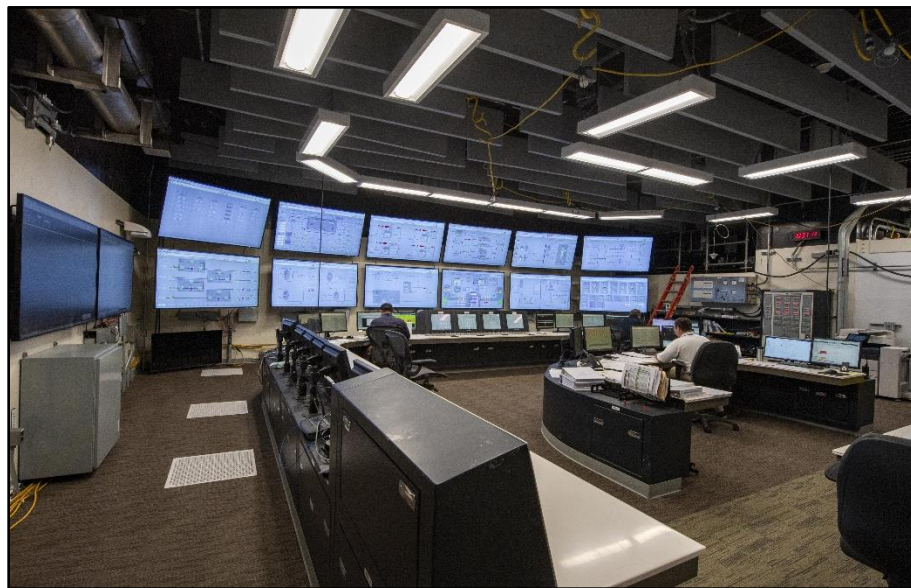
Unit 4 Main Control Room
