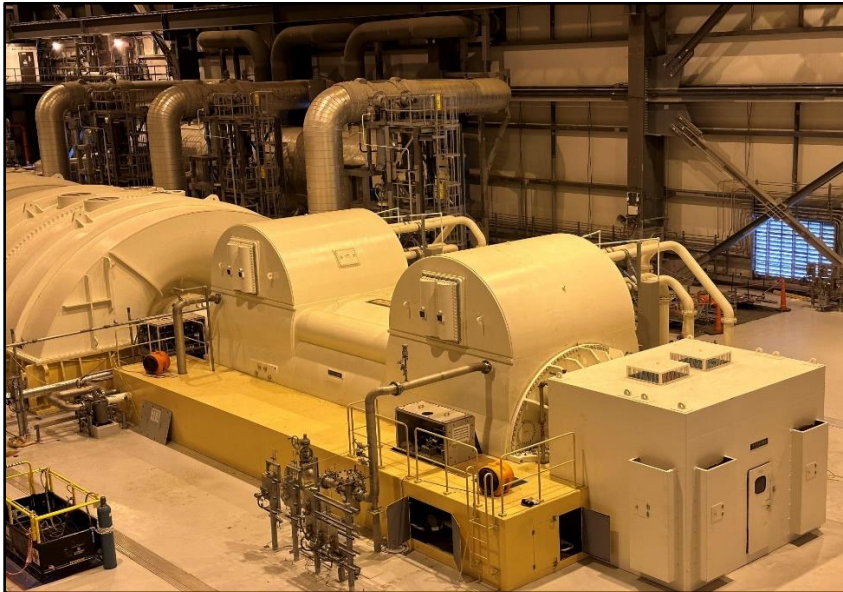
Unit 3 Planned Maintenance Outage
