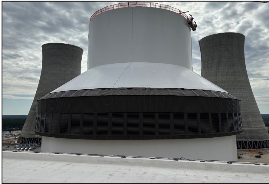
Unit 4 Passive Containment Cooling Water Storage Tank
