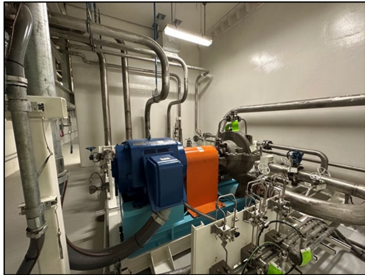
Unit 3 Spent Fuel Pool Cooling Pump
