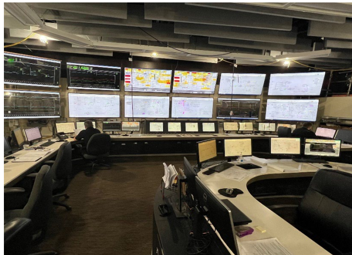
Unit 4 Main Control Room
