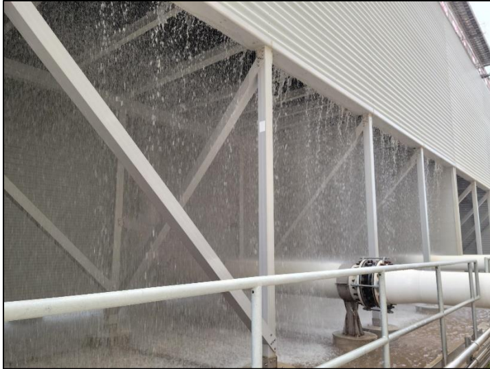
Unit 4 SWS Cooling Tower
