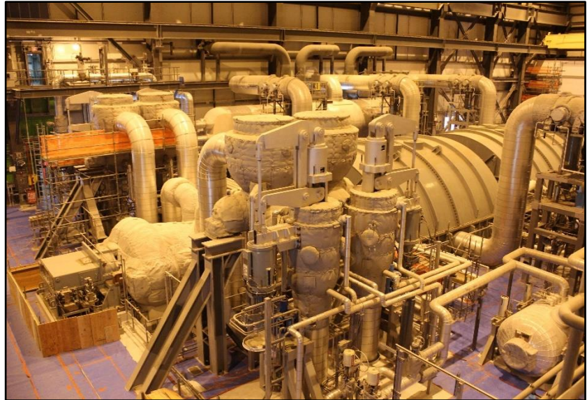
Unit 3 Steam Turbine
