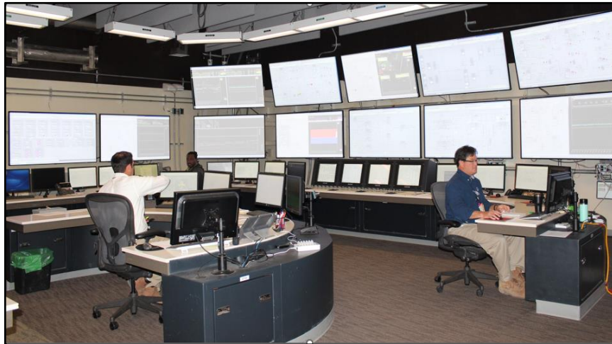
Unit 3 Main Control Room
