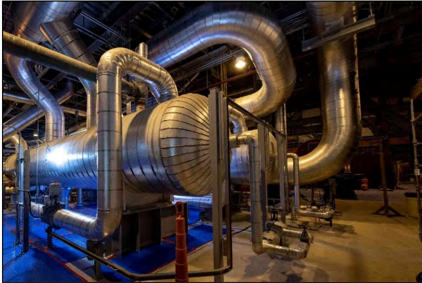
Piping Insulation inside the Unit 3 Turbine Building
