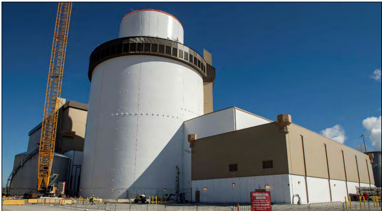
Unit 3 Nuclear and Turbine Islands
